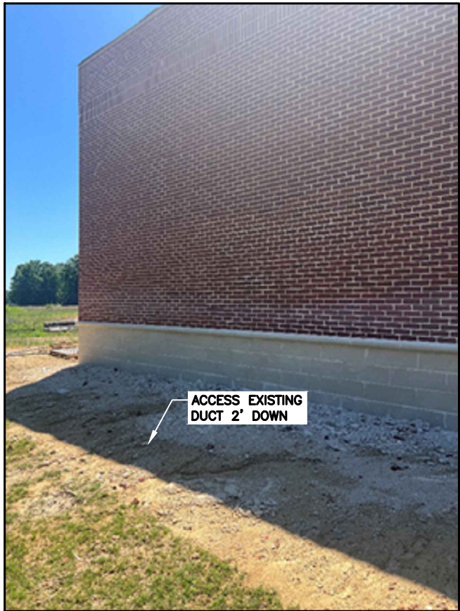
@2+91 ACCESS EXISTING DUCT AT A 45° ANGLE. USE 1.00" DUCT TO INTERCEPT. MAKE SURE TO SEAL THE DUCT.
